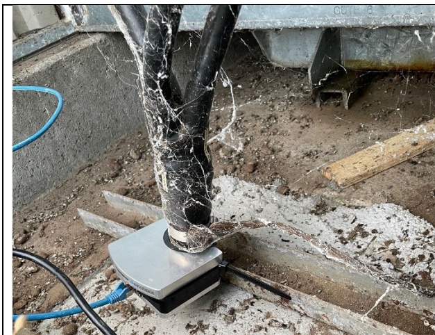
Installation at cable entry – only current measurement
