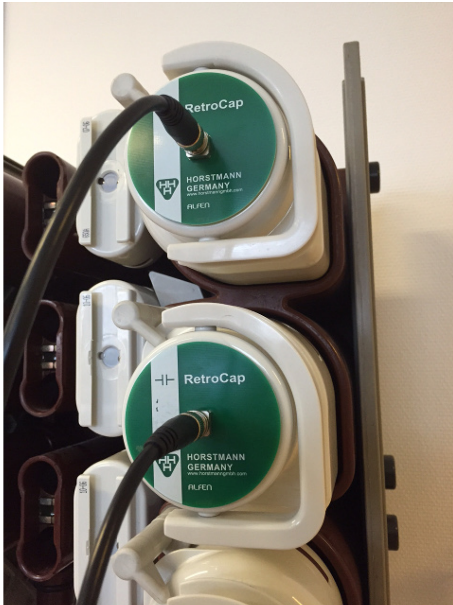
Figure 20: Horstmann RetroCaps mounted on Magnefix switchgear.
