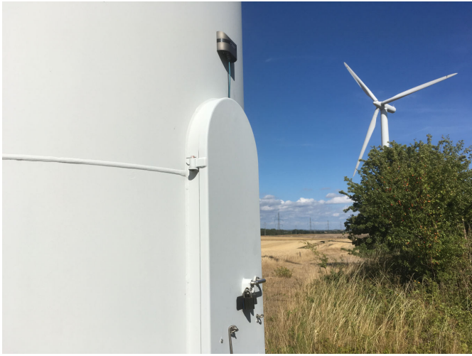
Sensor mounted above wind turbine door
