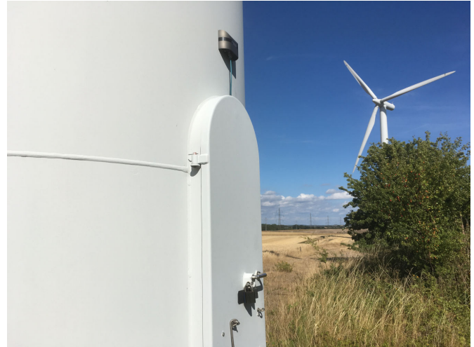
Sensor mounted above wind turbine door
