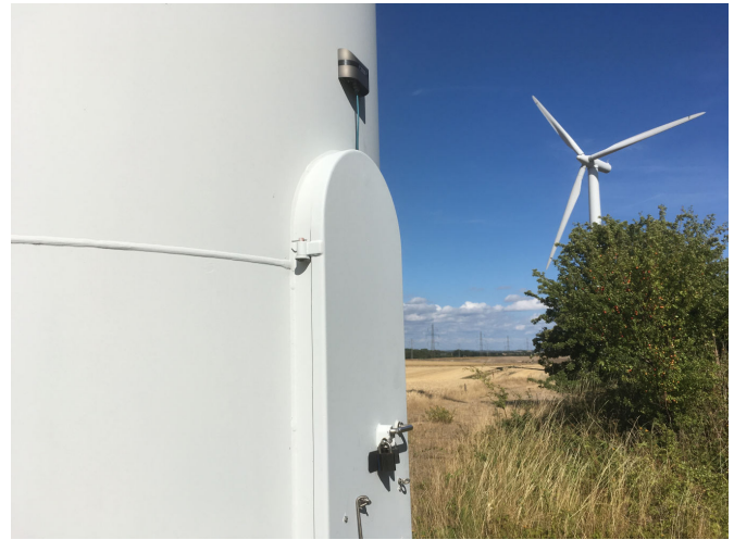
Sensor mounted above wind turbine door
