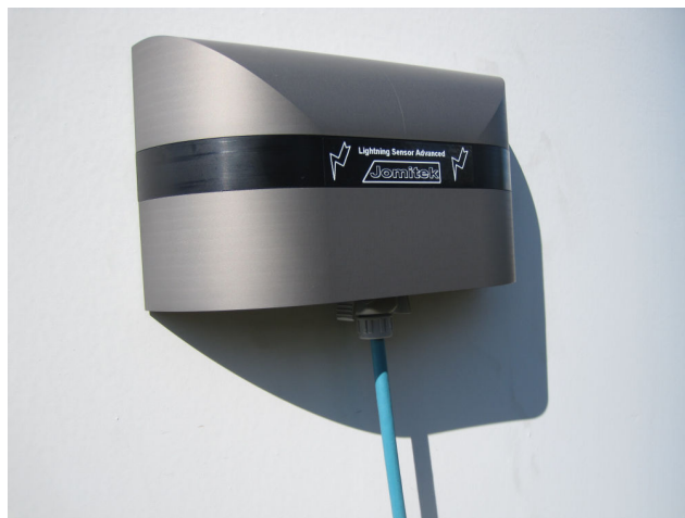
Lightning Sensor & Analyzer including the IP67 rated Ethernet cable connection.
