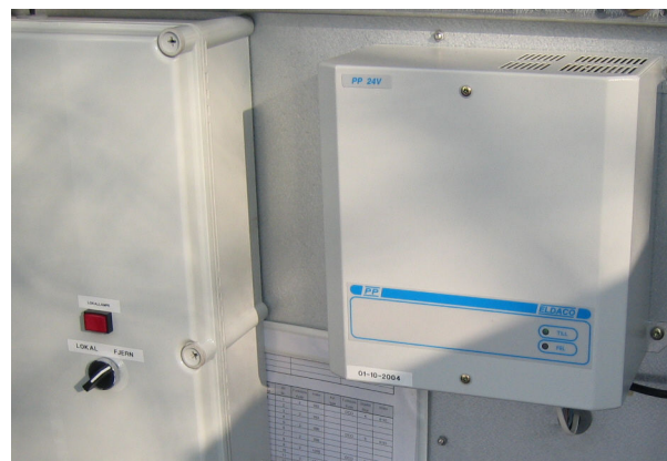
Figure 1, 24V supply in substation (HEF- Denmark)
